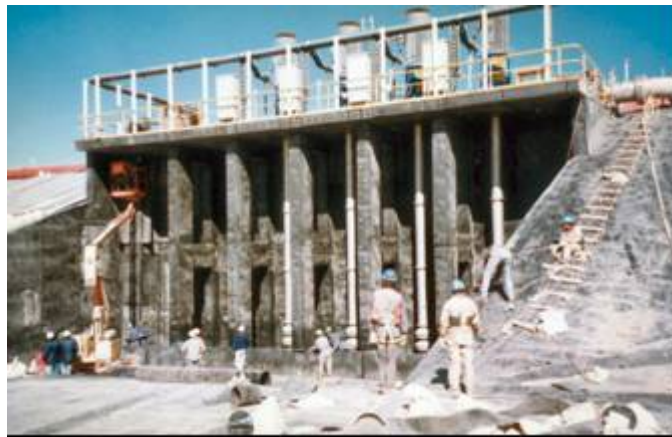
Figure 7. View of the Pump Station in PLS pond.
