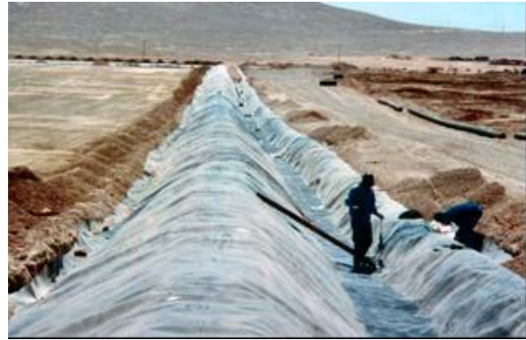
Figure 9. View of the collector channel in a unlined heap leach.
