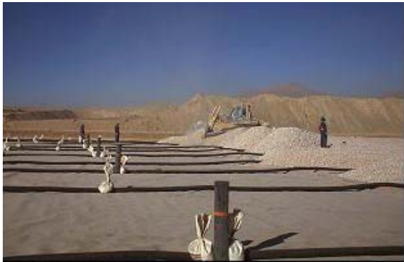
Figure 8. View of drainage systems in a heap leach.
