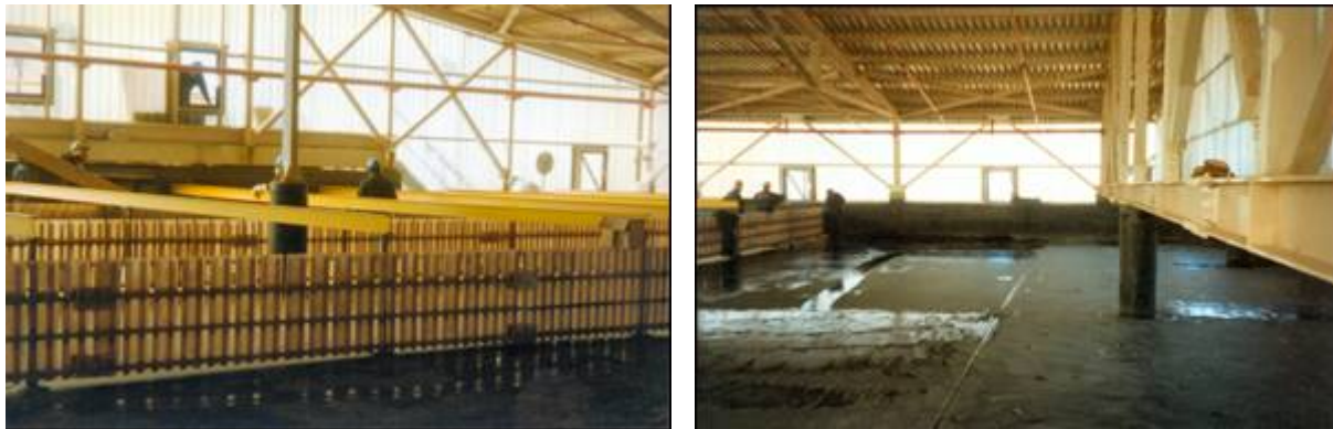
Figures 5 & 6. Two different views inside the Solvent Extraction area. The walls and the floors are lined with studded HDPE liner.
