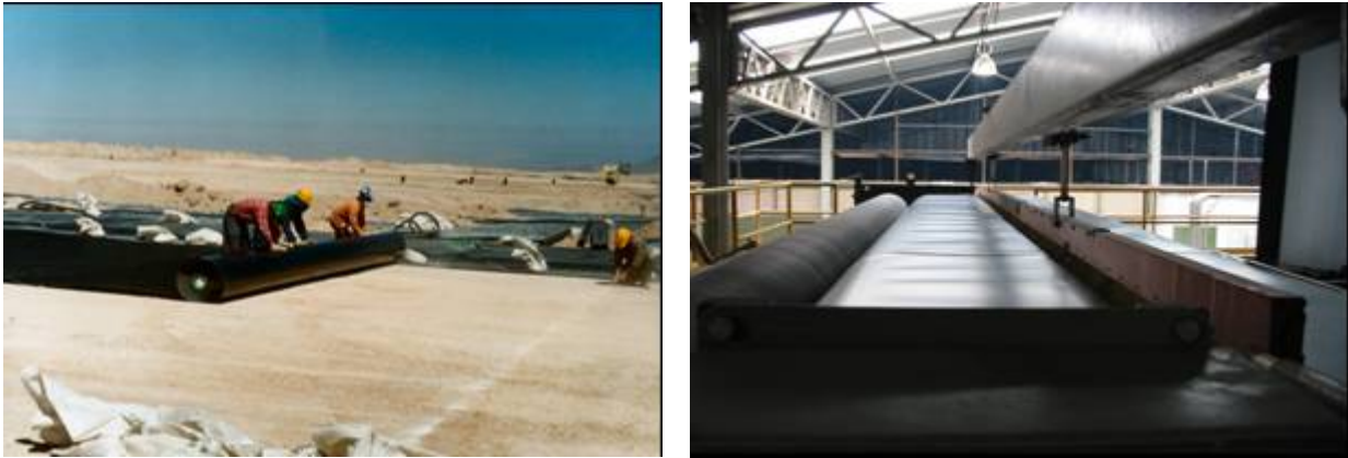
Figures 12 & 13. The spark test detector (right) can't help when the liner is not properly installed or deployed (left).
