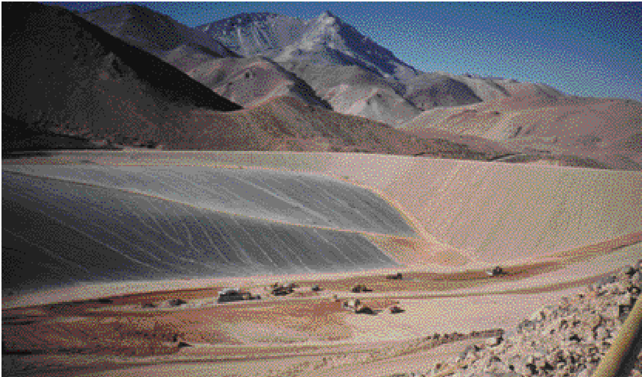
Lining an impoundment and dam at a gold mine located over 14,000 feet in elevation in the Andes Mountains of Chile, South America. High sloping canyon walls formed the sides of the impoundment, with a rock-filled dam located downstream. The dam is 200 ft high and is constructed from mine overburden rock. A dual geomembrane liner and geonet leak-collection system provided a seal to inhibit seepage through the porous rock fill.
